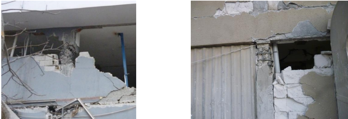
Figure 9. Shear damage on the captive columns
