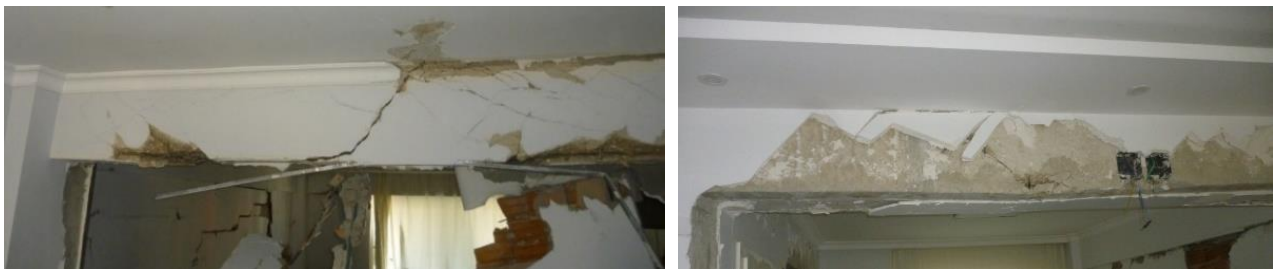
Figure 7. Shear damage near the mid span of the beam
