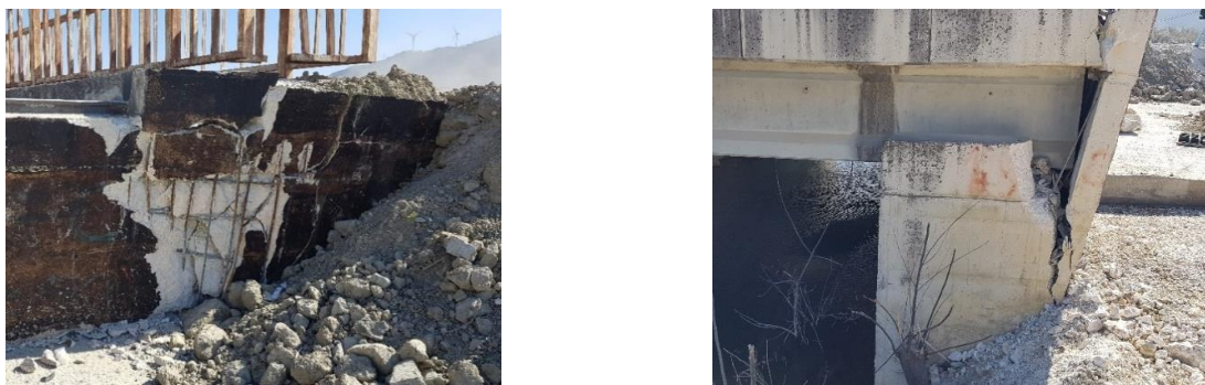
Figure 18. Back wall damages caused by pounding between the abutment and superstructure in the longitudinal direction
