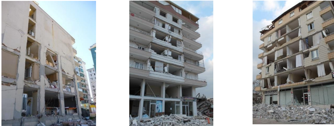
Figure 6. Out-of-plane tipping of exterior infill walls in ribbed slab systems
