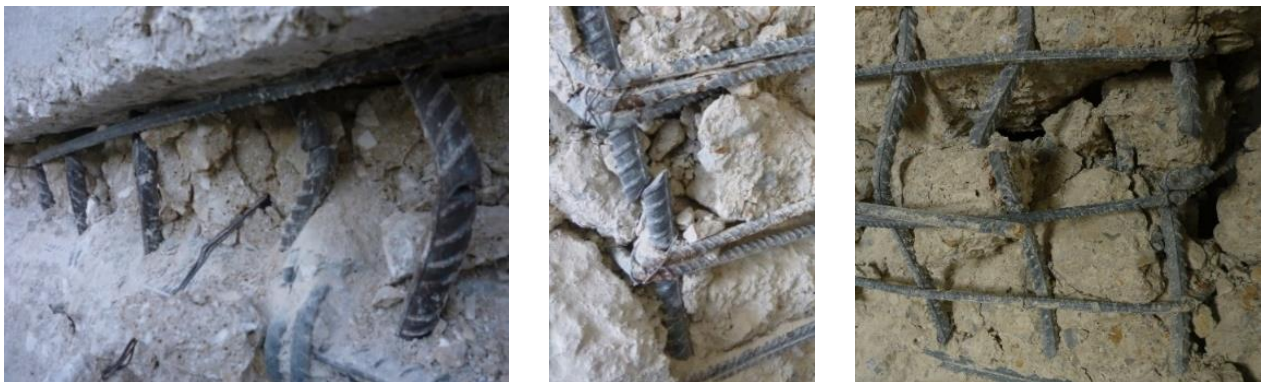
Figure 16. Fracture of reinforcement rebars
