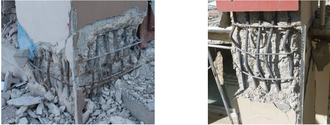
Figure 10. Large spacing between stirrups
