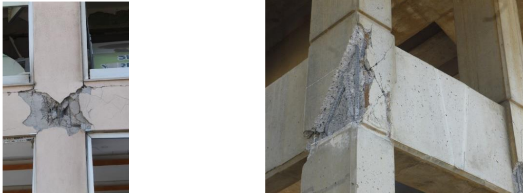
Figure 14. Not using transverse reinforcement in beam-column joints
