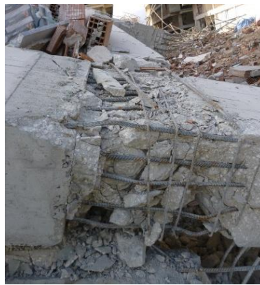
Figure 15. Lack of cross-ties in beam-column joints
