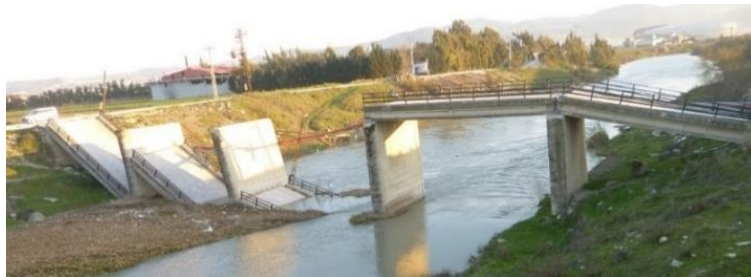
Figure 20. The unseating of superstructure of a bridge, which is out-of-service on the Hatay Hospital road, Coord: 36.27212, 36.20774
