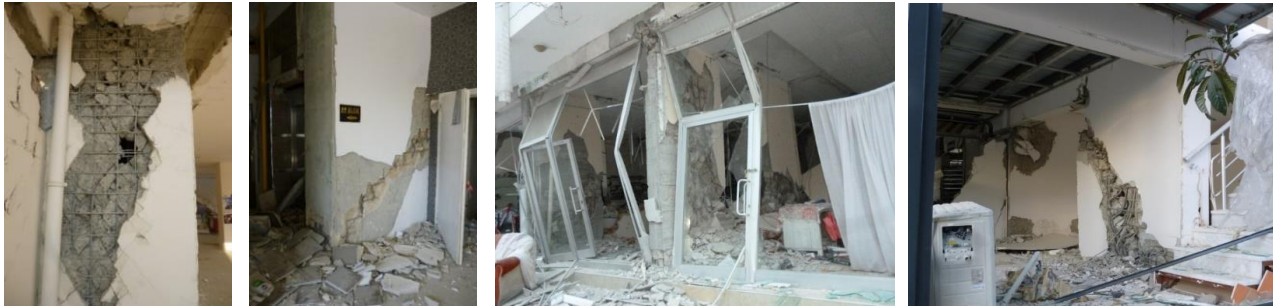
Figure 5. Shear failure of shear walls
