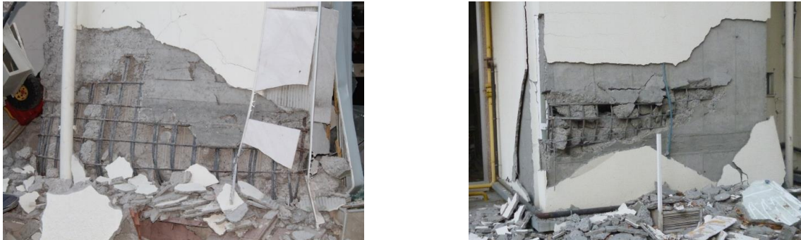
Figure 13. Lack of crossties in the shear wall
