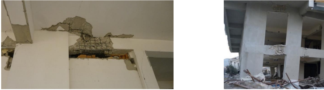
Figure 8. Shear damage of short beams
