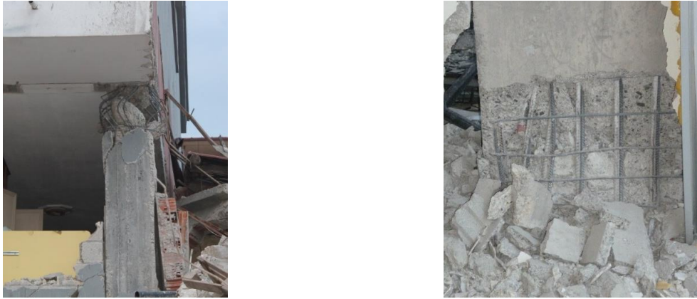
Figure 12. Lack of stirrups or crossties in the confinement zones
