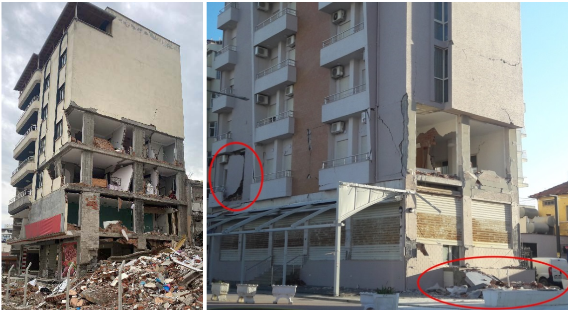
Figure 1. Damage and OOP collapse of infills in RC buildings: left (Turkey 2023), right (Albania 2019)
