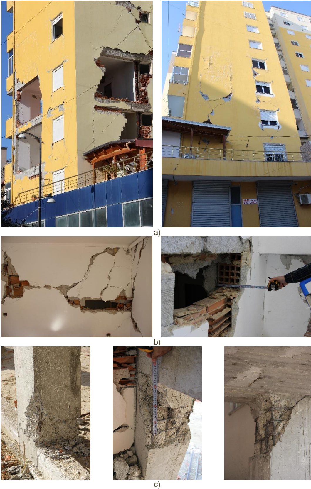
Figure 1. Damage to URM infilled RC frame buildings after M_w=6.4 ( I_{EMS}=VIII ) 2019 Durrës, Albania earthquake: a) view of the damaged building; b) very heavy damage or destruction of URM infill walls; c) slight or moderate damage of RC frames (Grünthal et al., 1998; Chungwook et al., 2020; Abrahamczyk et al., 2022a, 2022b)
