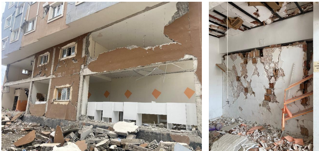
Figure 5. Damage of infill walls made of hollow concrete blocks and hollow clay blocks.
