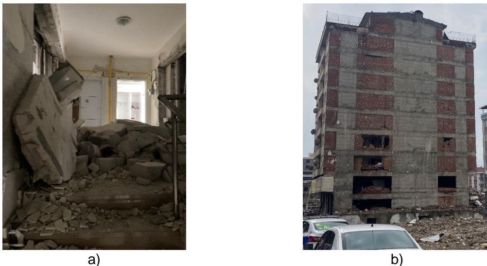
Figure 6. a) AAC infill damage blocking escape routes at stairwells and b) damage and collapse of infill walls on the lower stories
