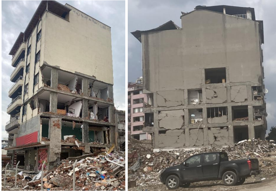
Figure 1. Damage and OOP collapse of infills in RC buildings without structural damage (Turkey 2023)
