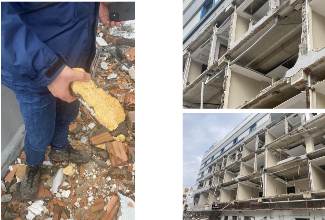
Figure 4. Hospital in Iskenderun: Damage and collapse of infills
