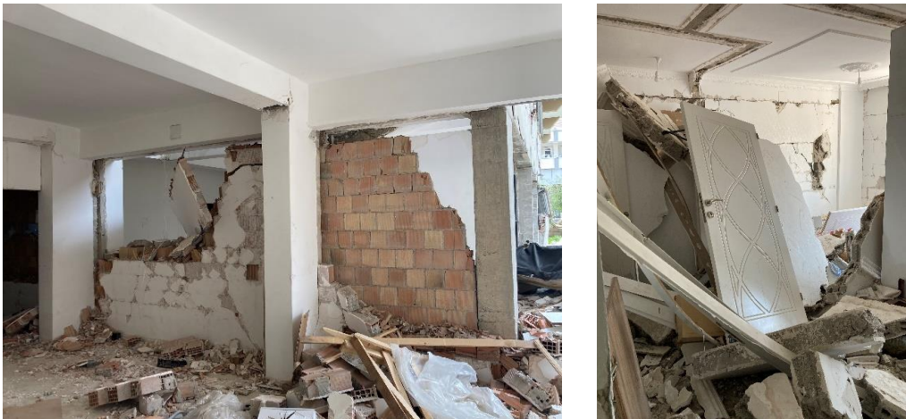
Figure 7. Infill damage inside the buildings
