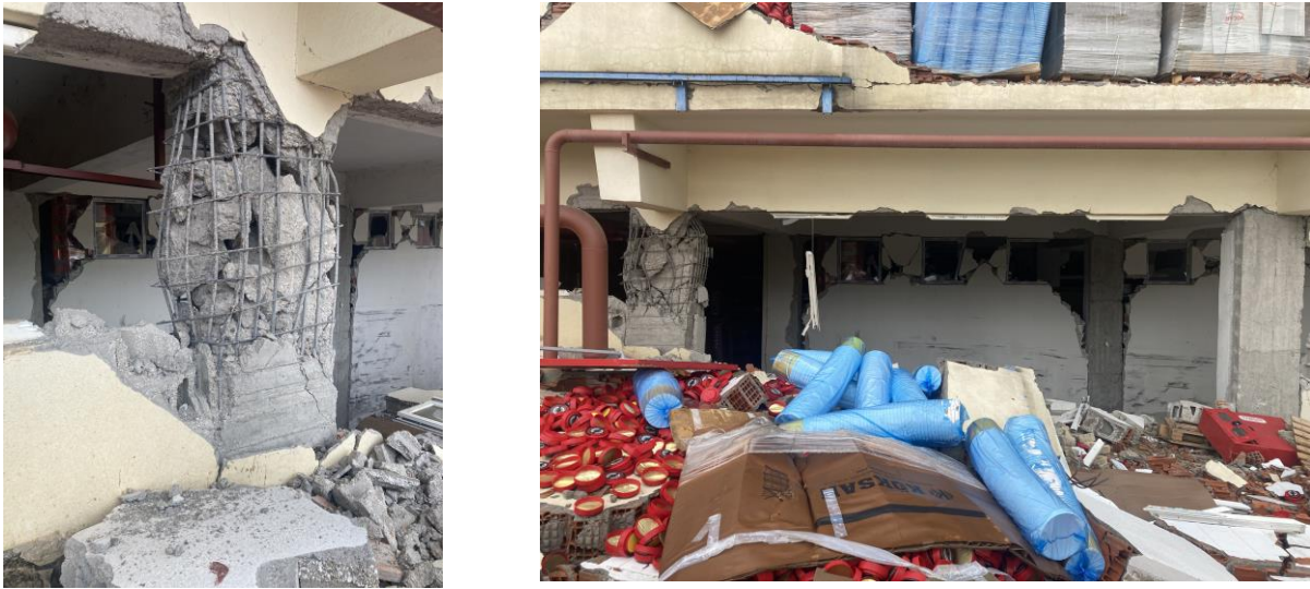
Figure 3. "Short column" effect due to interaction between RC column and partial height infill
