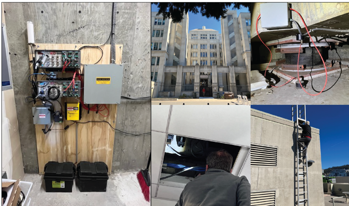
Figure 7. 2022 upgrade to digitizer at Berkeley City Hall, California
